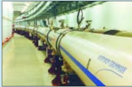
Figure 13. A section of the RHIC accelerator that creates colliding beams of relativistic heavy ions at BNL.
