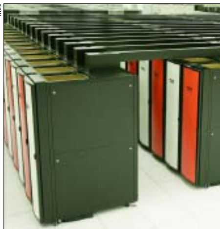
Figure 1. In April 2007, the ORNL Leadership Computing Facility increased the computing power of Jaguar, a Cray XT-3 computing system, to 119 teraflops, making it the most powerful open scientific system in the world.
